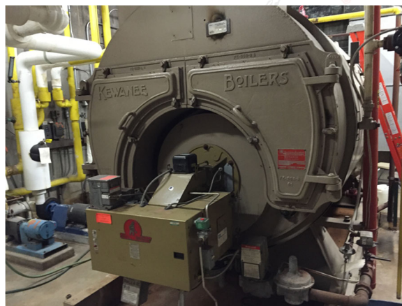
Boiler nearing end of useful life
