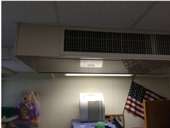
Fan coil and dehumidifier - needs HVAC update
