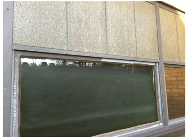
Window and Kalwall - needs replacement
