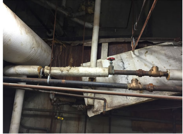
Mechanical ductwork needs to be replaced
