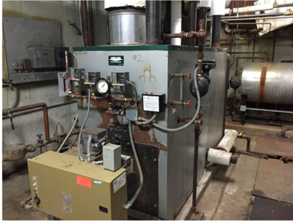
Boilers past useful life—need replacement
